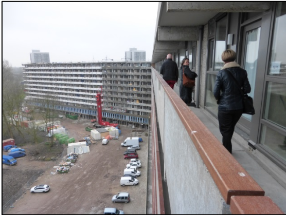
Fig.6 – De Flat, Amsterdam – The City of Amsterdam is enabling 500 private homebuilders to invest in a large refurbished ‘shell’ block of apartments
